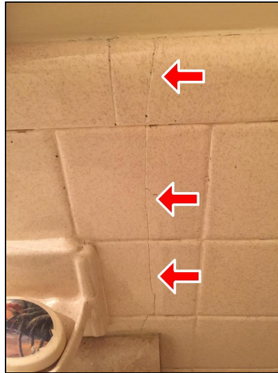
4.1 Item 1(Picture) Cracked Tile
