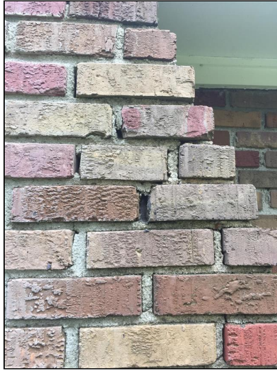
1.2 Item 2(Picture) Missing Mortar Joints
