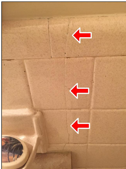
4.1 Item 1(Picture) Cracked Tile
