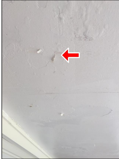
2.0 Item 2(Picture) Peeling Paint
