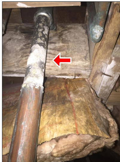
6.0 Item 2(Picture) Leaking Waste Piping
