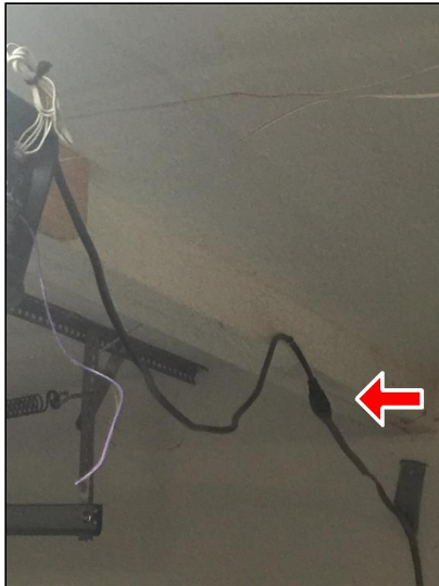
3.5 Item 1(Picture) Garage Door Opener Extension Cord
