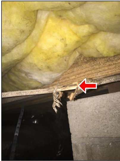
7.2 Item 1(Picture) Frayed Wiring
