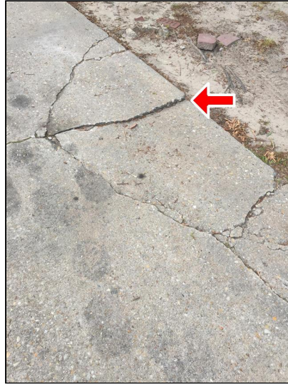
2.4 Item 1(Picture) Driveway Settlement
