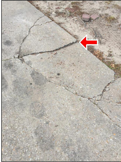
2.4 Item 1(Picture) Driveway Settlement
