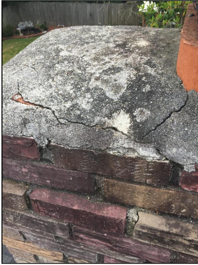
1.2 Item 1(Picture) Cracked Chimney Crown
