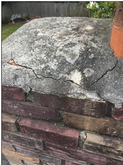
1.2 Item 1(Picture) Cracked Chimney Crown
