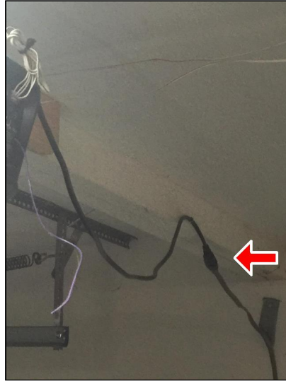
3.5 Item 1(Picture) Garage Door Opener Extension Cord
