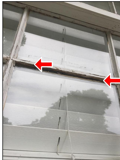
2.2 Item 1(Picture) Missing Window Glazing
