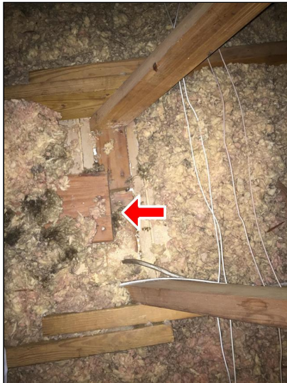
9.0 Item 1(Picture) Missing Insulation
