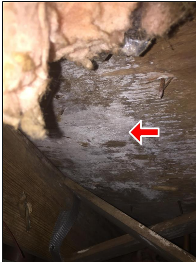
5.0 Item 1(Picture) Possible Fungal Growth
