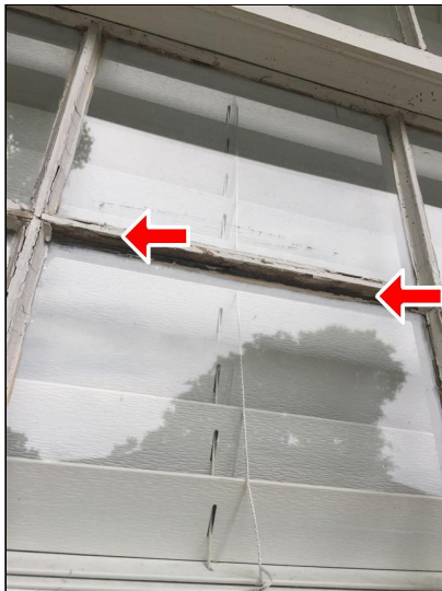
2.2 Item 1(Picture) Missing Window Glazing
