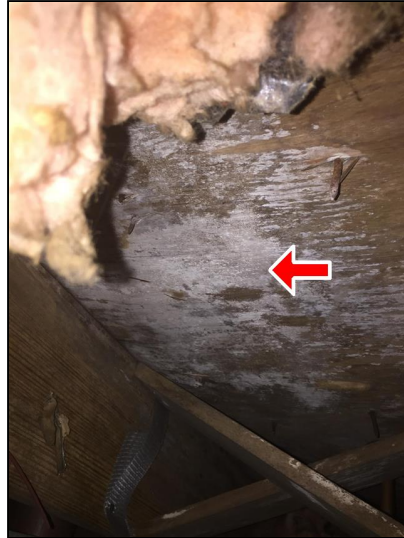
5.0 Item 1(Picture) Possible Fungal Growth
