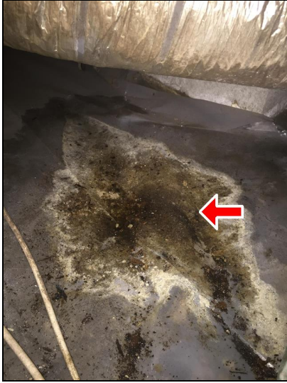
6.0 Item 1(Picture) Standing Water From Waste Pipe Leak
