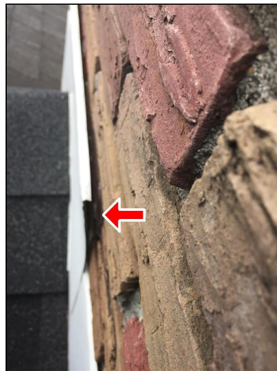
1.1 Item 1(Picture) Loose Chimney Flashing
