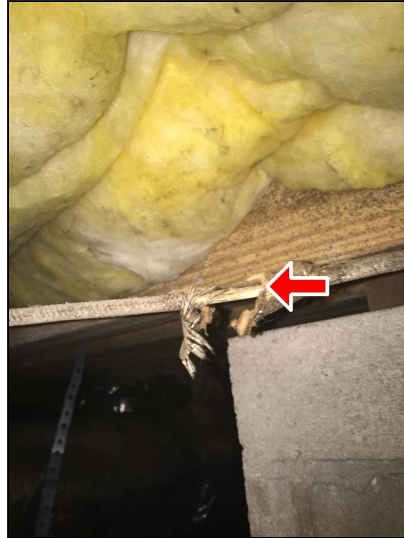
7.2 Item 1(Picture) Frayed Wiring
