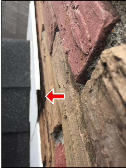
1.1 Item 1(Picture) Loose Chimney Flashing
