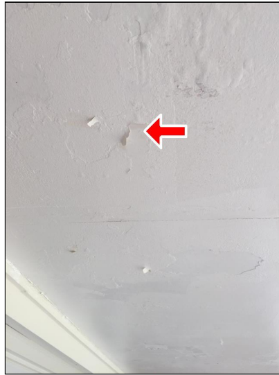
2.0 Item 2(Picture) Peeling Paint
