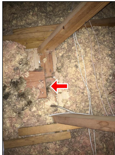
9.0 Item 1(Picture) Missing Insulation
