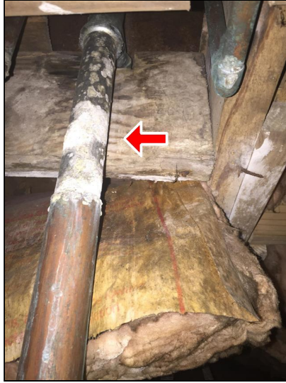
6.0 Item 2(Picture) Leaking Waste Piping
