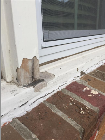
2.0 Item 1(Picture) Peeling Paint
