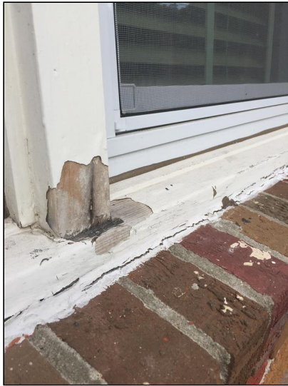
2.0 Item 1(Picture) Peeling Paint
